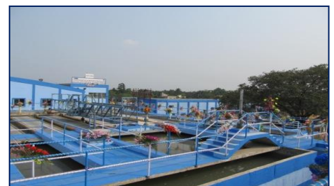
32 MGD WTP at Madhyamgram
