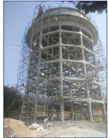
Over Head Reservoir
